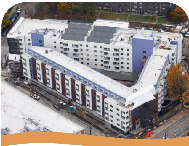
Construction progress of the Red Cedar apartment building located in Yesler from 201X to 2018; the building will open in 2019.
