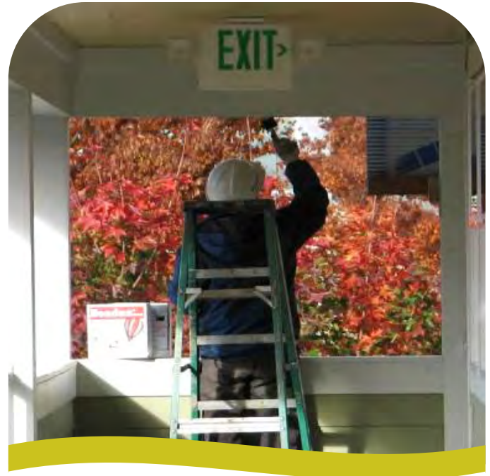
Repairing the exterior of an SHA-owned apartment complex located in south Seattle.
