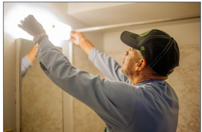
An SHA employee doing preventative maintenance work on an empty unit in Yesler Terrace.
